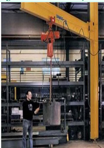
Fig. 5: Wall mounted jib crane
